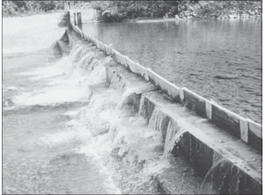
This diversion dam on Peshastin Creek blocks salmon and bull trout from migrating up stream.
